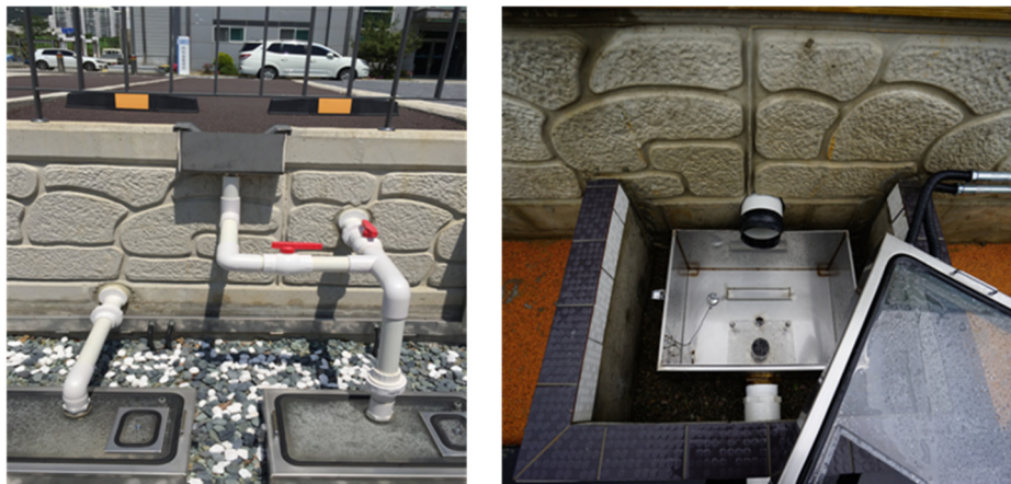
Figure 5. Monitoring system for parking lot(left) and architectural (right)
