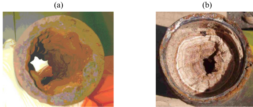
Figure 2. Blockages with irregular shapes in practical water supply pipelines, (a) encrustation and biofouling in a cast iron pipeline (James and Shahzad, 2003), and (b) clogged section in a seawater pipeline ( http://pureelementswater.net/ ).
