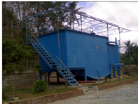
Figure 2. Water treatment installation.
