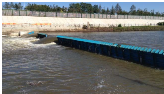
Figure 5. Gate lowering of Aodong hydraulic elevator dam.
